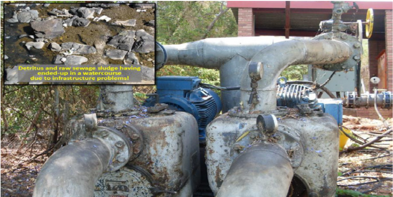
Vandalism, ageing infrastructure and insufficient maintenance of sewage infrastructure
